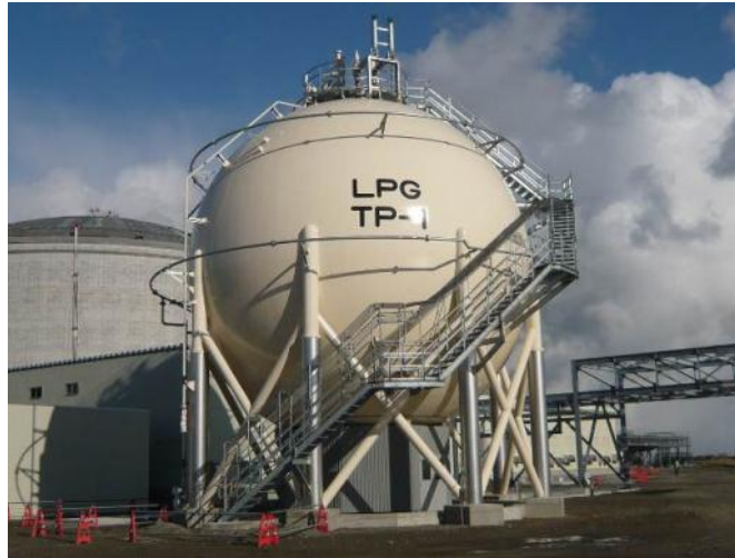
LPG storage tank
