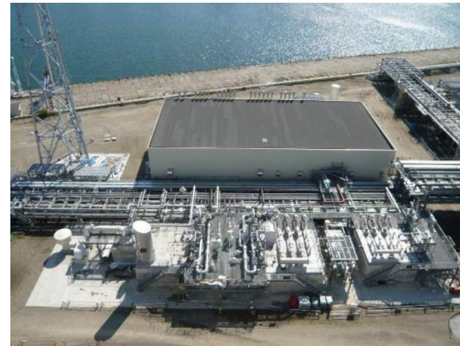
Vaporizer(this side) Building for utility. (other side )
